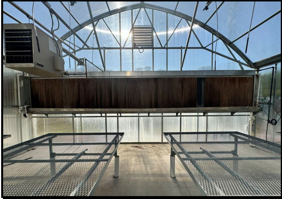
View of cooling system
