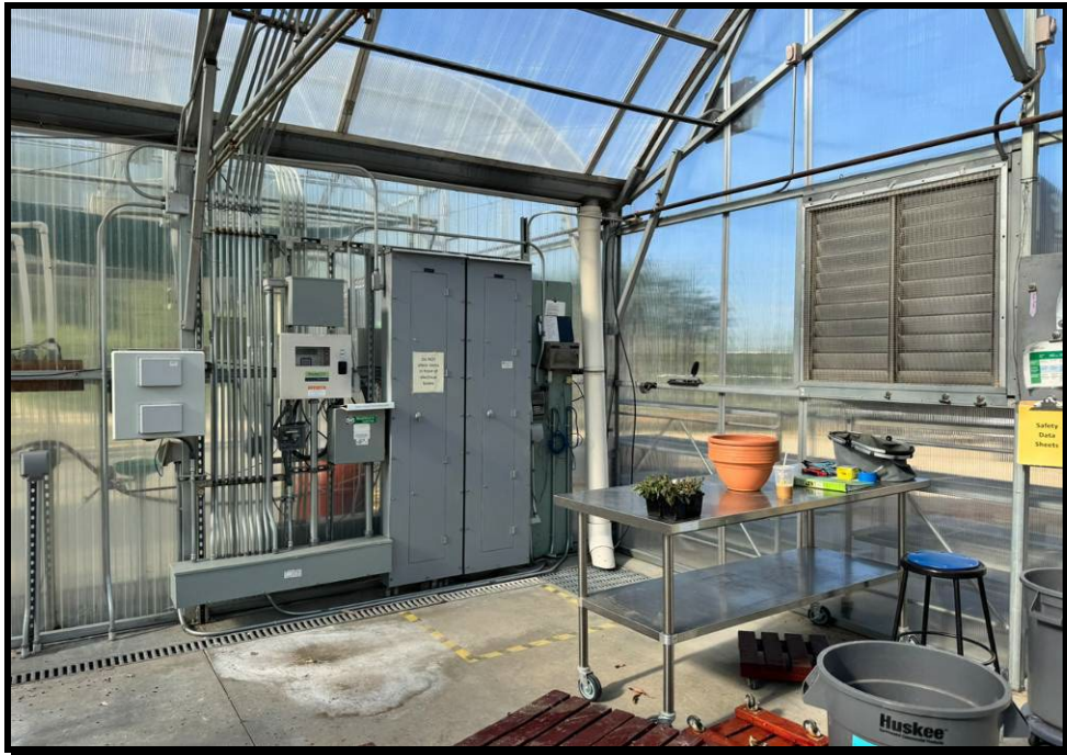
View of electrical for both greenhouses
