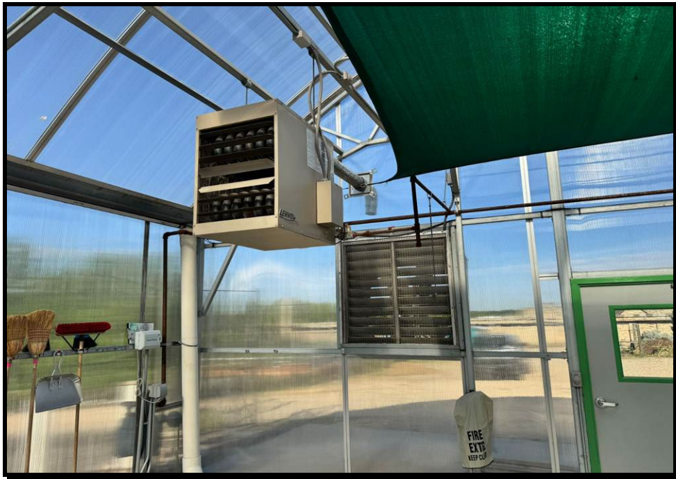
View of space heater
